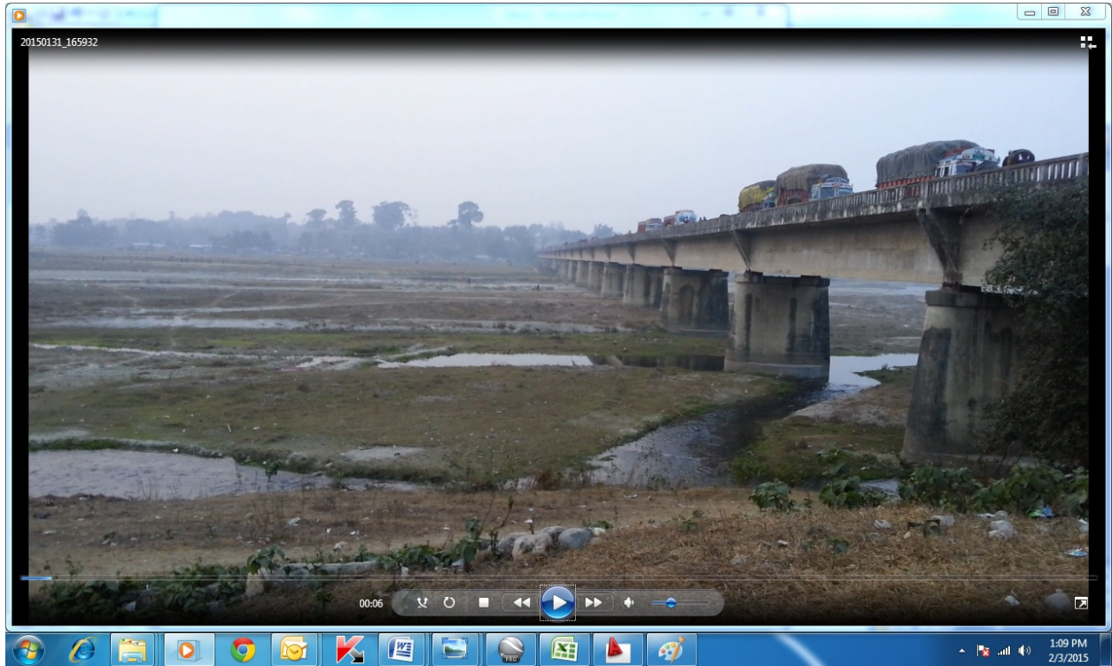
Photo-3: General elevation of the bridge from downstream and Combined interlaced channels and piers vulnerable to concentrated flow line
